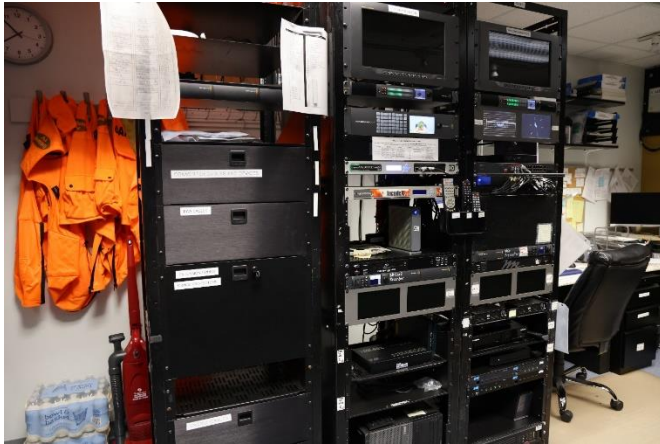
Oakland TV booth equipment racks, August 1
